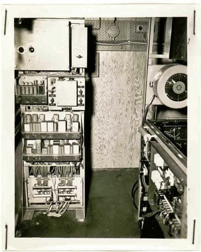
Neg. No DB 8001 Dispo: L HQ Dest Photo'g Arndt E Dept: HMCS "BRUNSWICK/ ASDIC GEAR INSTALLED IN HMCS "BRUNSWICKER".
