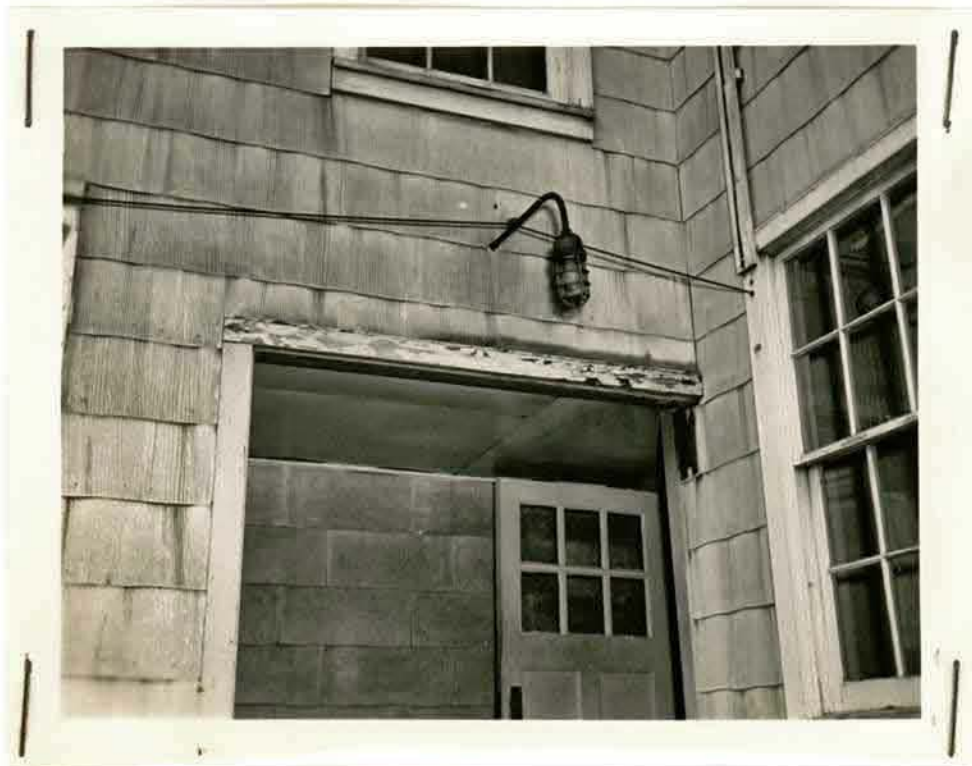
Neg. No DB 8004 Dispo: L HQ Dest [ ] Photo: Arndt E. Dep: HMCS "BRUNSWICKER" Cap: CONDITION OF PAINT on outside walls of HMCS "BRUNSWICKER".
