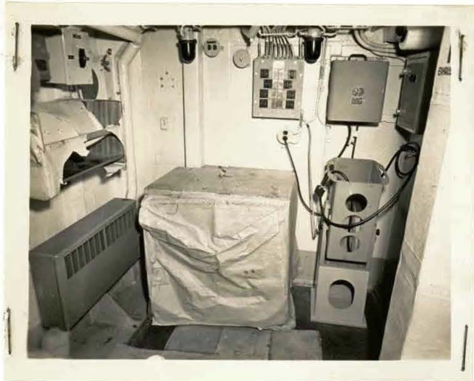
Neg. No. DB 7912 Dispo: HQ Dest Photo: Carroll CANFLAGLANT Dept. ST. ANTHONY Caption: IN DRYDOCK. View of Chart Room.
