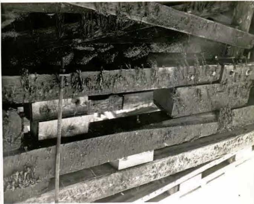
Neg. No. DB 8706 Dispo: L HQ Dest Photo's Carroll Dept. Boatshed Caption Damaged jetty View showing hole through and metal bar for support.
