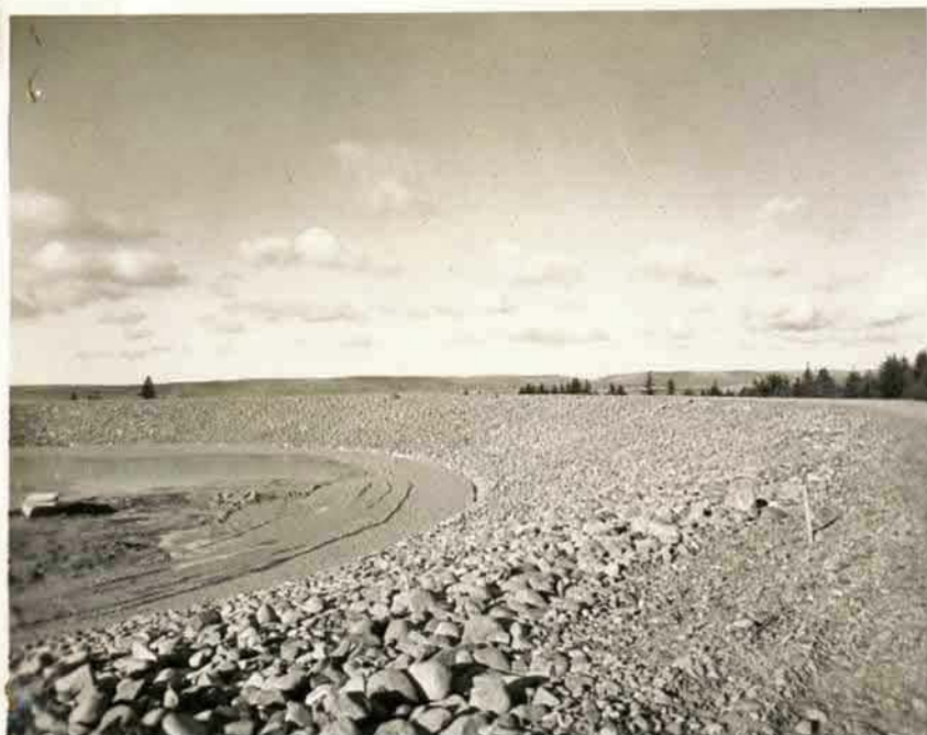
Neg. No. DB 9982 Dispo. L. / HQ. / Dest.. Photo 'g. Carroll. Dept. Maintenance Caption. Progress shots. View showing reservoir.
