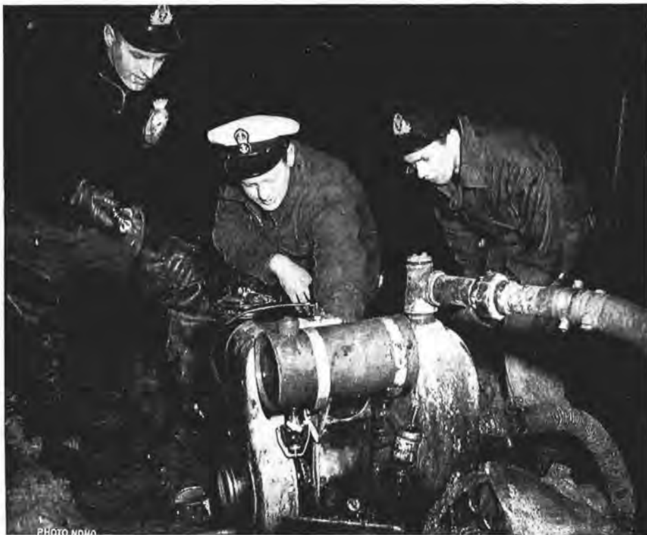
Working with a suction pump behind a dike in one of the flooded areas of Winnipeg are Lieut. K. A. Laidlaw, RCN(R), Ret'd., PO James Harris and Lieut. D. A. MacDonald, RCN(R), all of HMCS "Chippawa." (O-1408-31)
