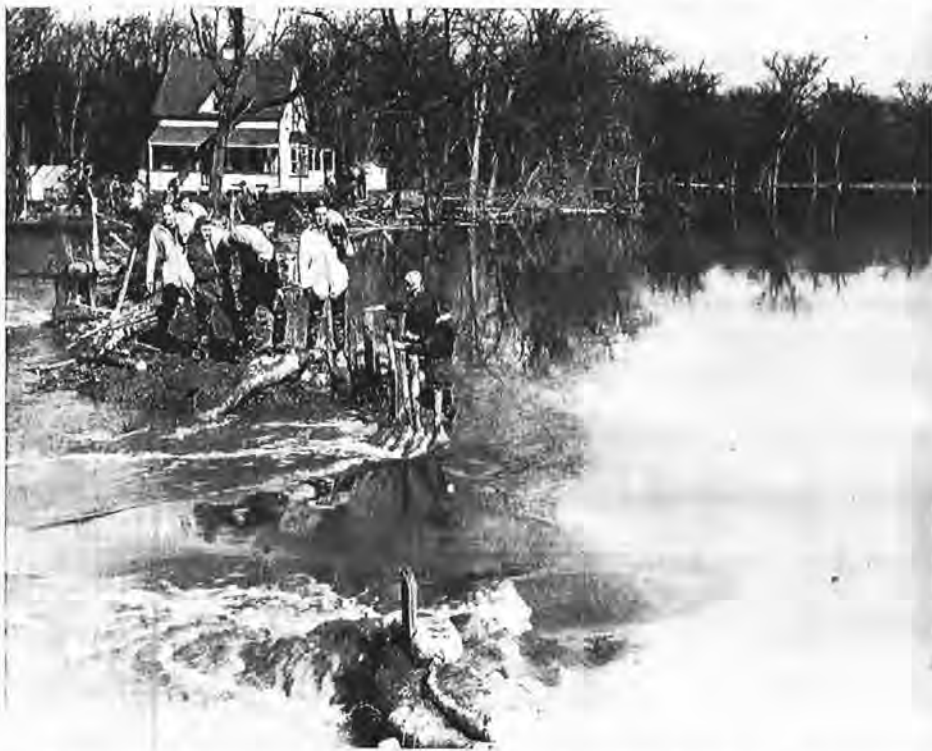
Soldiers from Prairie Command repair a breach in a dyke of the Assiniboine River two miles east of Poplar Point. The Army's assistance was requested to close the break, which was causing heavy inundation of farmland in the area. The soldiers worked throughout Saturday afternoon until darkness forced a halt. They then returned to the area Easter Sunday morning to complete the task, which was their first flood assignment this year. This is the third successive year that troops have been used in this area to repair dykes. (Canadian Army Photo)
