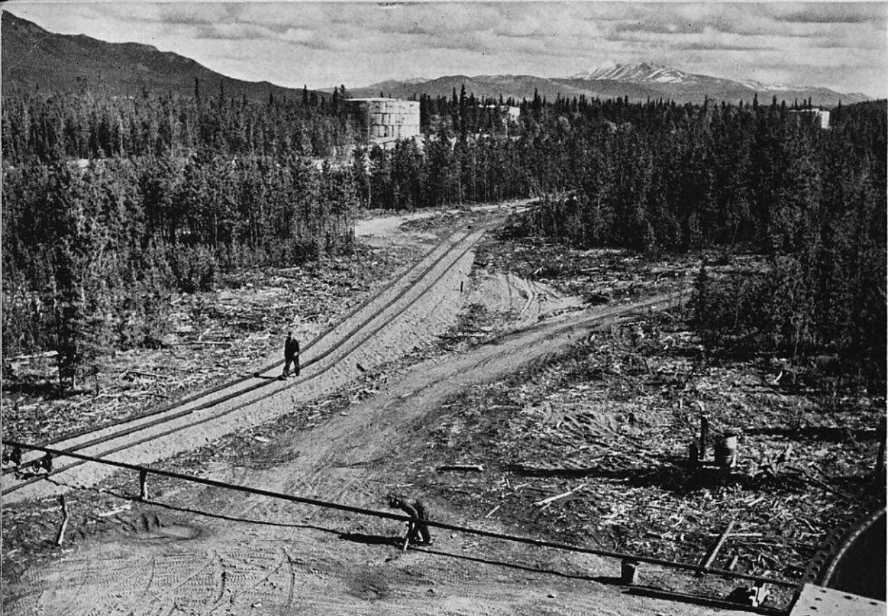
Long lines of pipe criss-cross at a tank farm somewhere along the Canol Project.
