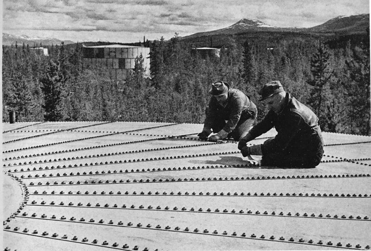
Tightening bolts on top of huge storage tank at large tank farm somewhere along Canol pipeline. Tanks are shipped in sections and subsequently bolted together.
