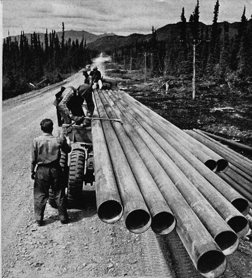
Along the Alaska Highway roar huge trucks carrying seven-ton loads of pipe. Here a load of pipe is being dumped. Pipe layers and welders will take over from here.
