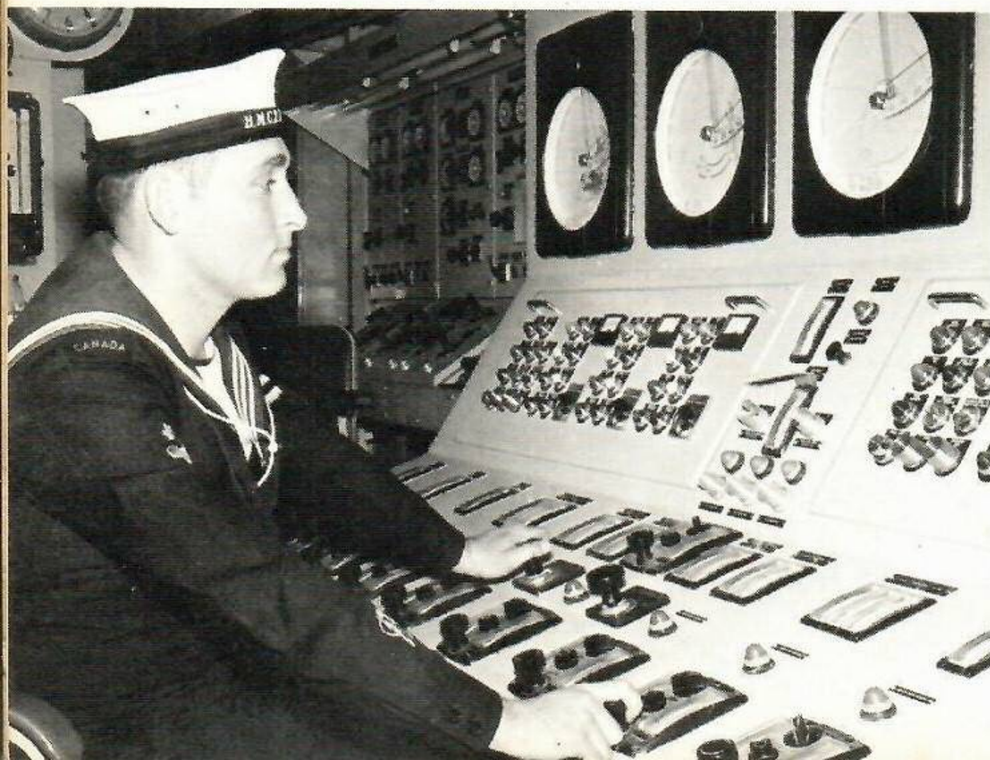
Machinery Control Room
