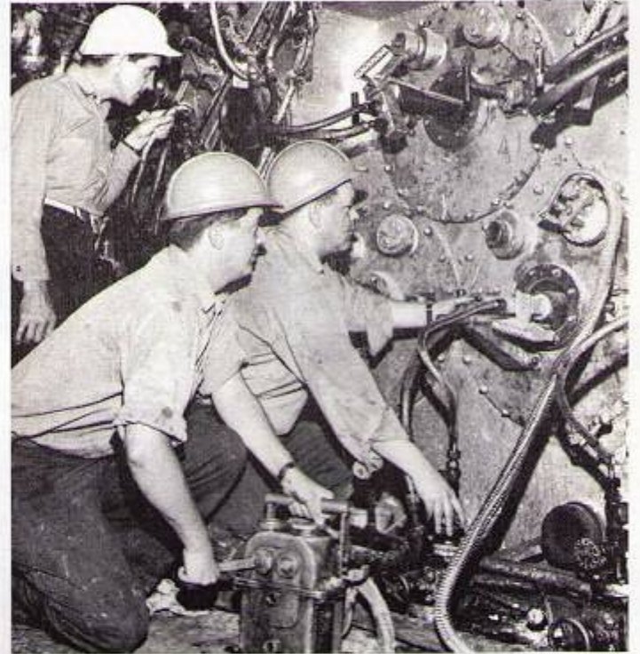
The end of the job was in sight when engineers flashed boilers for first time.
