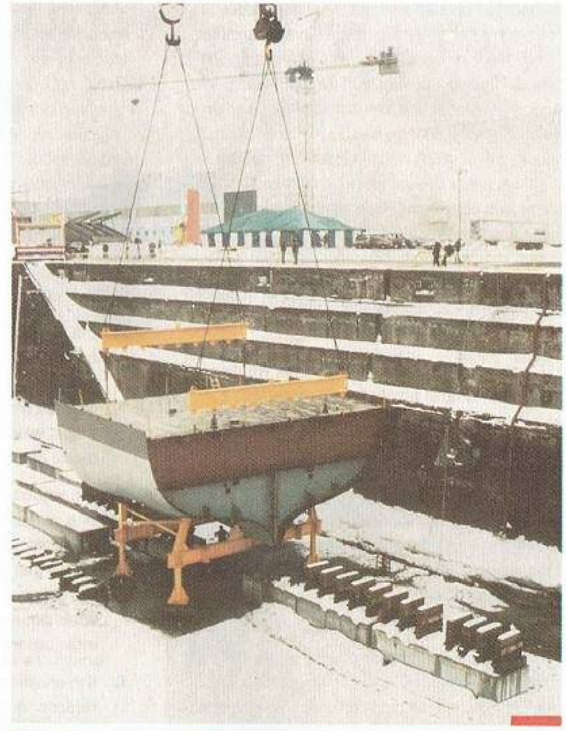
Erection of keel unit for CPF 01 in dock at Saint John Shipbuilding Ltd. on 19 March 1987
